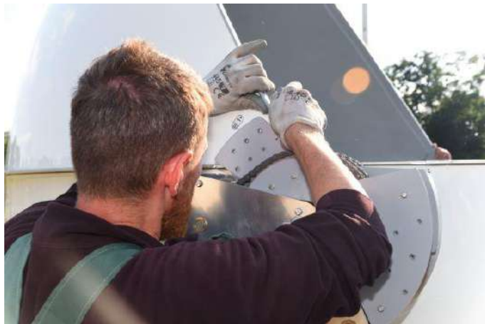
Figure. 40 – Shutter no. 1 in the handles.
